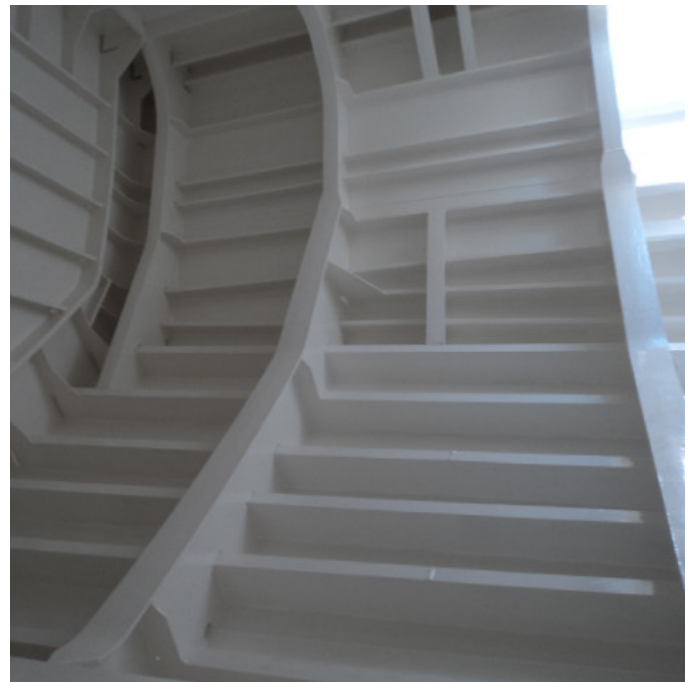
■ Apply 1 coat of 300 \mu of tar component, solvent free, heavy epoxy tank lining.
